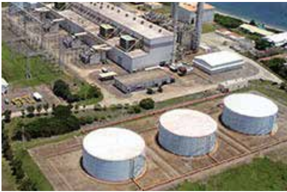
The 1,200MW Ilijan Natural Gas Power Plant under IPPA with SMEC is the largest electricity-generating facility in the Philippines that uses domestic fuel. [Photo courtesy of San Miguel Energy Corporation]
